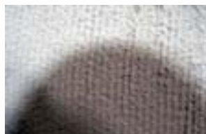
Thin set applied to the dry wall with a 1/8" "V" notched trowel
